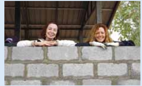
Kathleen Minck (left) and Cara Kramer, her roommate from Connecticut, are standing proudly behind the wall they just built.
